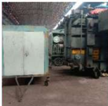
Filling dry air with Dry air generator
