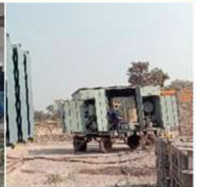
FILTRATION OF TRANSFORMERS
