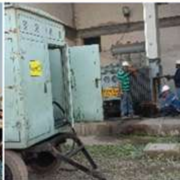
Transformer oil filtration
